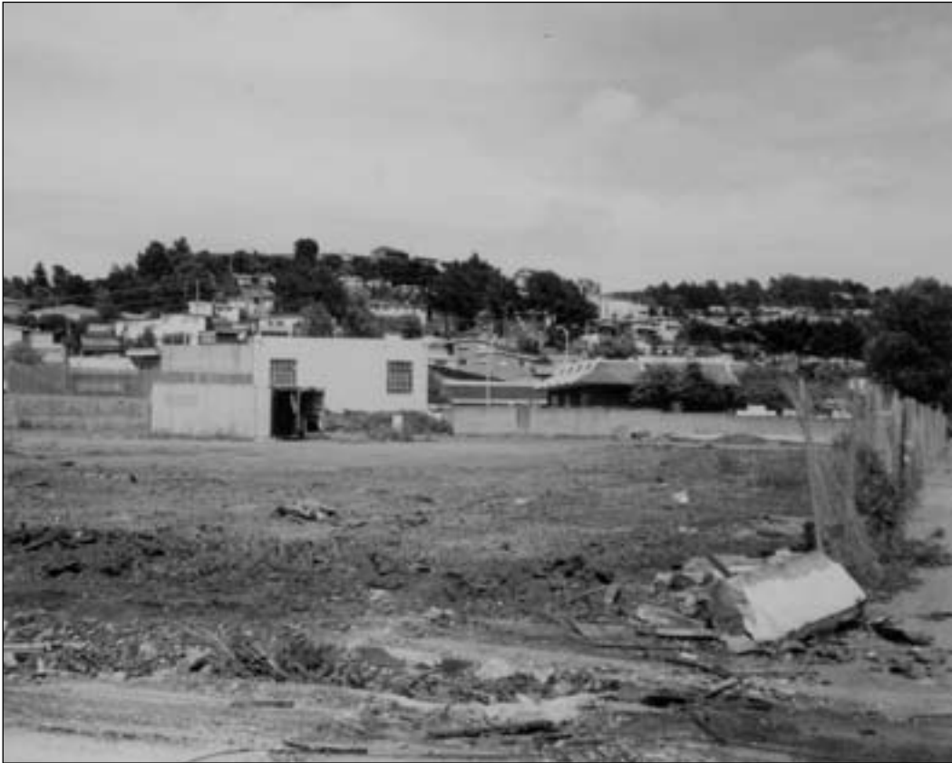
The end of the line in 1992 for the Japanese nurseries in El Cerrito. Between San Pablo Avenue and the Eastshore Freeway, everything (except a few buildings facing San Pablo Avenue) from Wall Avenue north through the Adachi property is being demolished to make way for Home Depot. The sidewalk of Wall Avenue is just visible on the right. ECHS collection, courtesy of the Hocking family.
